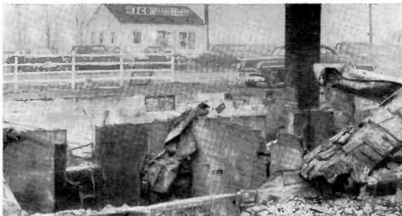
Smoke-blackened interior of KICD, gutted by fire on Easter Sunday.
